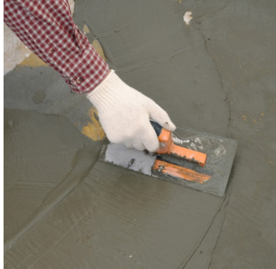
Feather-Edge Spalled & Pitted Concrete
